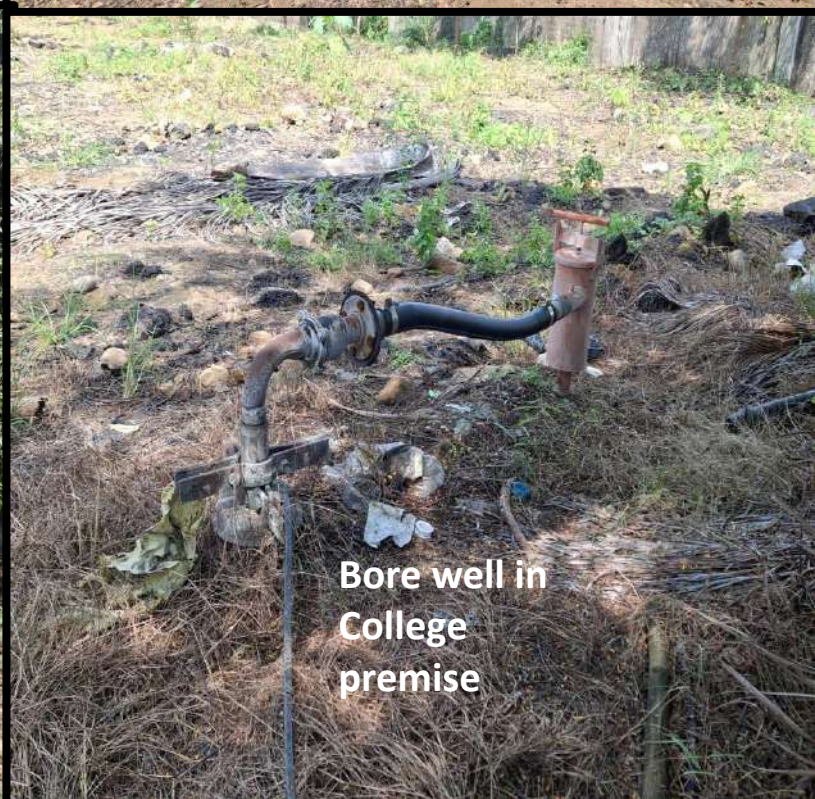
Rain Water Harvesting System
