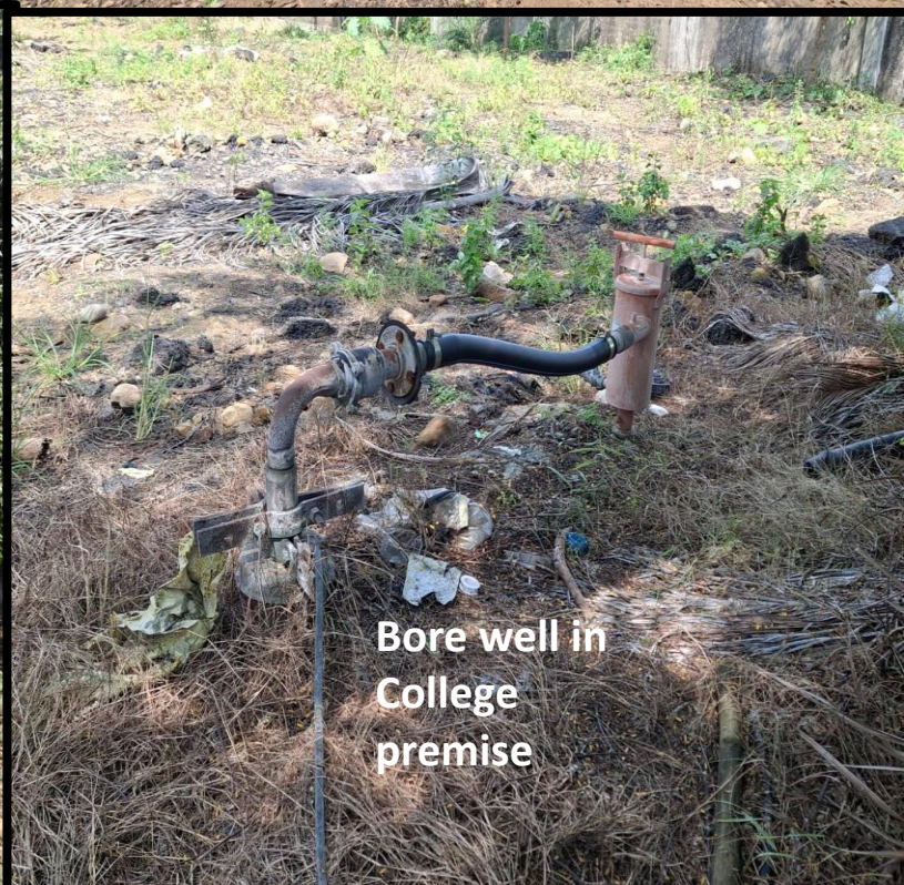
Rain Water Harvesting System
